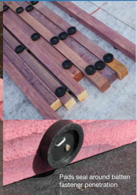
Elevated Battens allow free water flow off the roof
